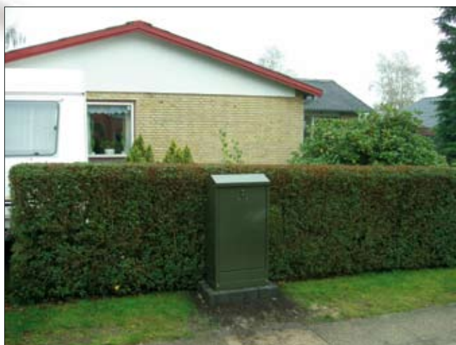
Installation in urban area
